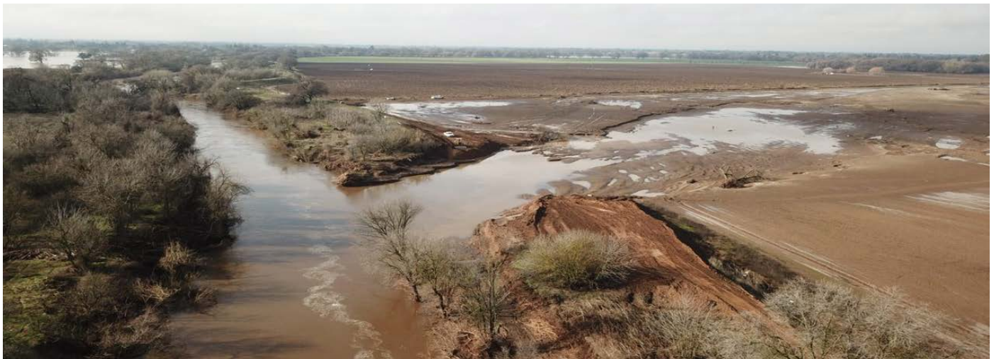
The photo shows the damage of a privately owned levee that did not qualify for FEMA funding.
